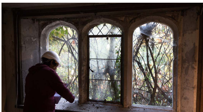
Vegetation coming through the mullion windows at St Andrews. November 2018
