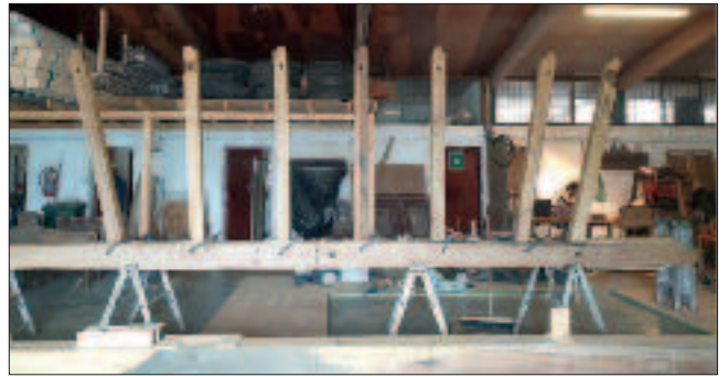
One sheer has its outriggers fitted. The four bolt holes for the clamps at the scarf can be seen. The second sheer is in the foreground. The outriggers will be cut to length when we have worked out how long they must be, and finished with fancy ogees.
