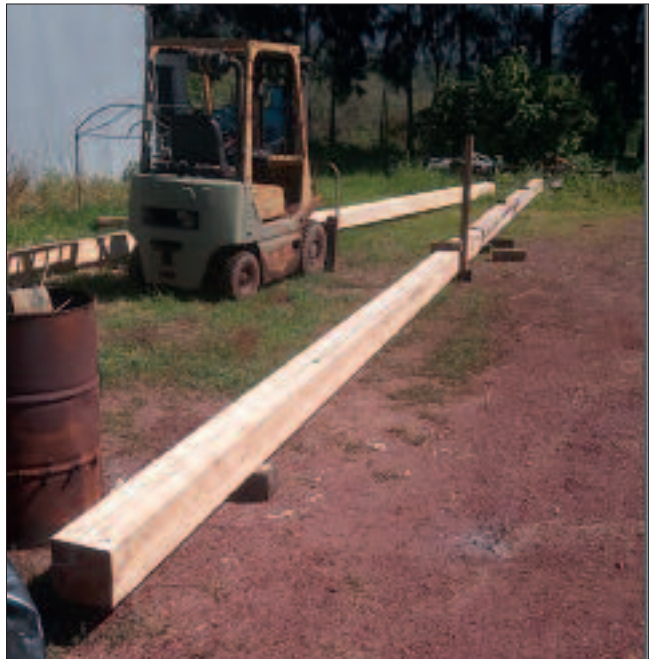
Two 8m beams laid end to end. Now they must be joined!
