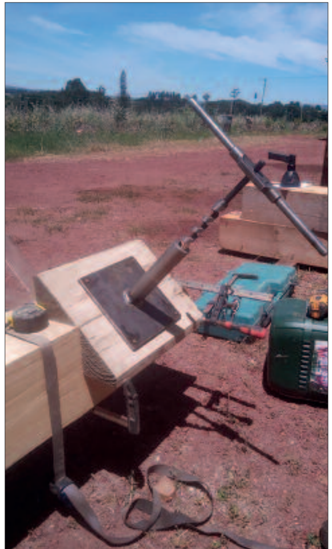
Each end of the long stretcher had to be drilled at 45 degrees for the bolt which attaches to the long brace which reaches down to the bottom of the tail pole at the back. Nervous moments, but it came out at the right place!
