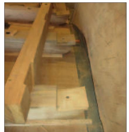
The dovetails have been modified in the sheers and Burgemeester so the front gable can lie over at 10 degrees.
