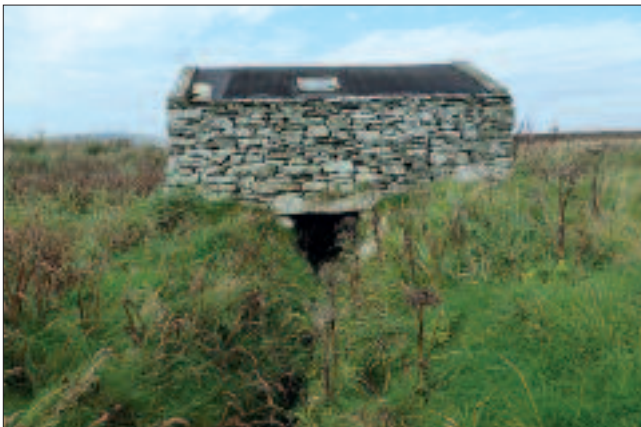
Fig. 4. The restored mill at Troswick, Dunrossness in 2011. The original roof has been replaced with a tarred felt covering. Picture courtesy of Derek Mayes
