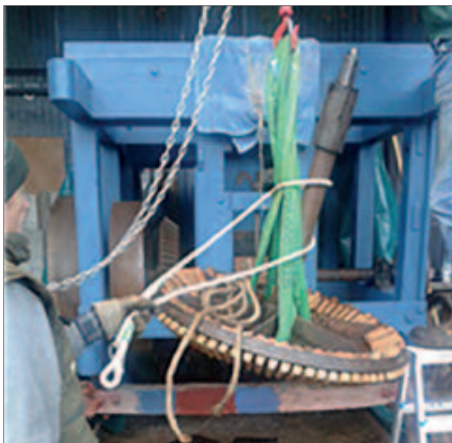
The crown wheel being lifted into place. Trial traces of Prussian Blue and Venetian Red are visible on the rear axle.
