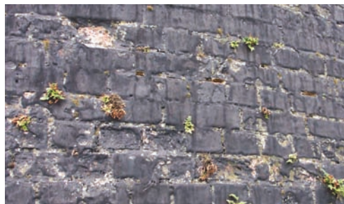
Broken-down tarred surface outside. Bricks spalling and vegetation starting to grow.
