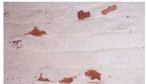
Limewashed surface inside showing effects of incipient damp penetration.
