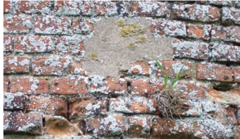
Untreated brick surface outside showing worn bricks, degraded pointing and crude cement repair. Vegetation starting to grow.
