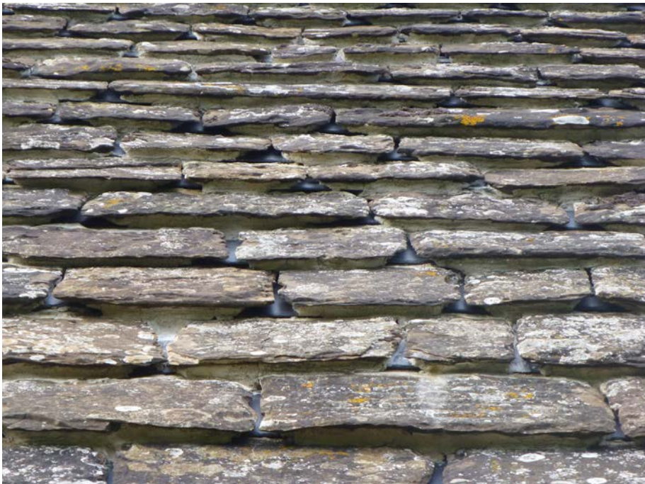
Horsham stone slate single-lapped with Welsh slate soakers at Botolphs Church, West Sussex (view angled to show technique). Photo credit: Rachel Morley.
