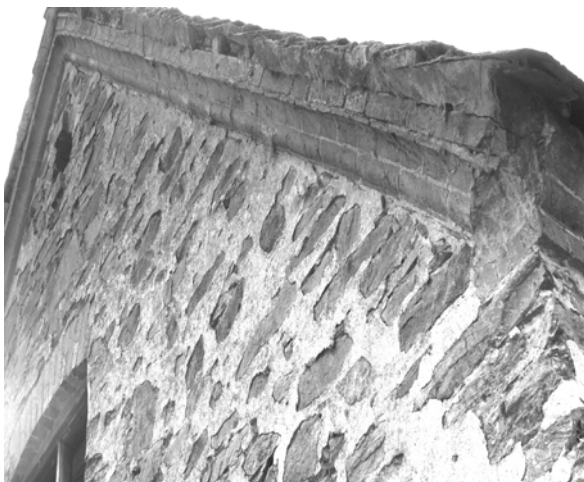
Figure 33 On later roofs verges were extended with decorative brickwork or terracotta. Terry Hughes
