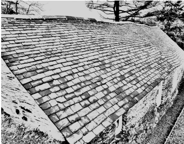
Figure 6b If undulations are only eased by the minimum to allow tight slating the roof's charm will be conserved. Terry Hughes
