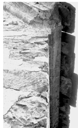
Figure 30 During the nineteenth century a large eaves overhang was formed by corbelling the wall head with decorative brickwork. Terry Hughes
