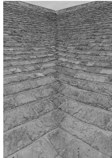
Figure 48 Collyweston valleys are always laced by laying a roughly square slates diagonally up the valley and turning the adjacent slates on each to butt up against them. Terry Hughes
