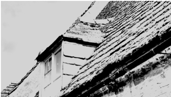
Figure 16a Where dormer ridges run into the main slating they are either swept up into the main slope or the junction is weathered with a lead saddle. Terry Hughes and Ray Harrison
