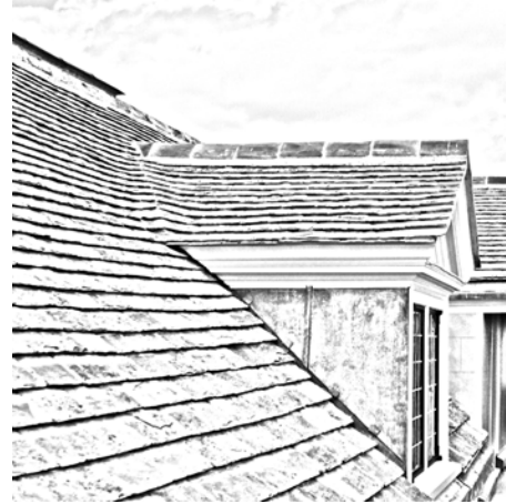
Figure 53 Dormer windows are common in Collyweston roofs and the full range of types - monopitch, gabled and hipped are common positioned below, breaking and above the eaves and in the roof slope.
