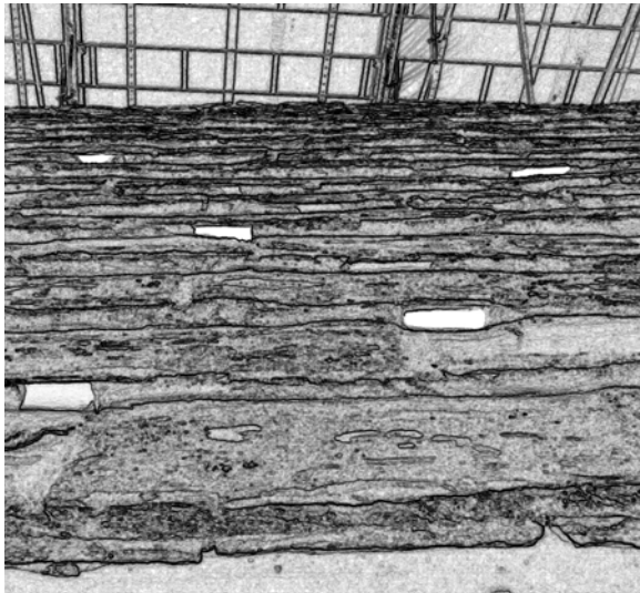
Figure 45 Fully bedded Collyweston slating is effectively sealed and cannot readily ventilate moisture from inside the roof. If ventilation is necessary small gaps can be left in the bedding. This also works as access for small bats. Terry Hughes
