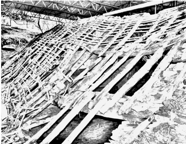
Figure 6a Movement of the roof structure may not require any correction or perhaps just stabilising. But if there are severe or abrupt undulations they can be impossible to slate over without the slates gapping even if small or narrow slates are used. In this case the undulations can be eased. Terry Hughes
