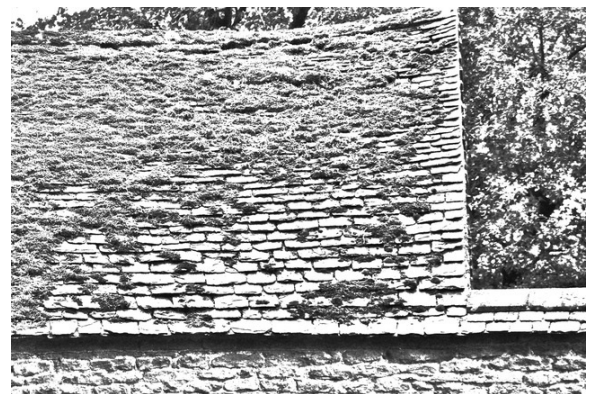
Figure 55 The roofscape of the Northampton area is confused because it includes original local stone slates, Collywestons and various Cotswold types. Many are not easily distinguished from each other without petrological analysis.
