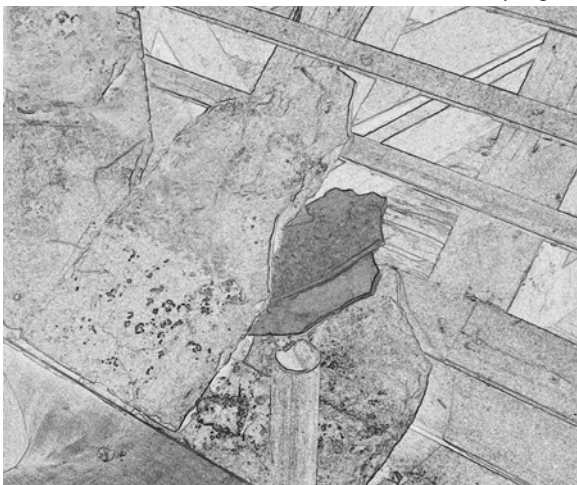
Figure 46 Shales or shadows are bedded in a small amount of mortar as the slates are laid to support their span from tail to head. Terry Hughes
