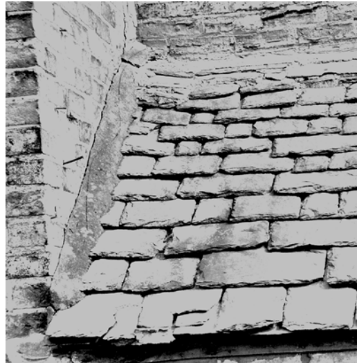
Figure 12 Before the availability or affordability of lead for soakers abutments were weathered with simple mortar flaunches. Terry Hughes
