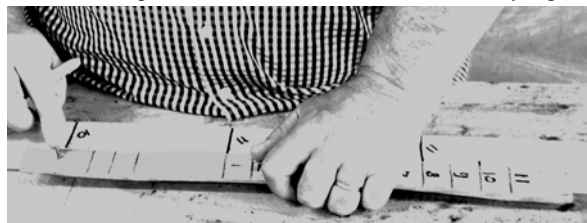
Figure 4: Gauging The stick is used to set out the margins and the lath gauges and these diminishes all the way up the roof. Terry Hughes
