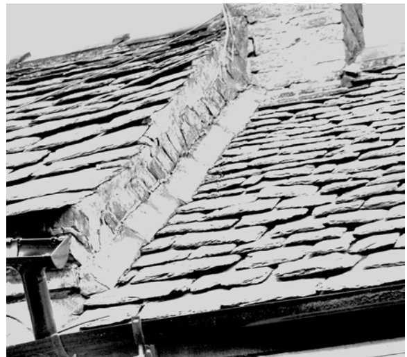
Figure 13 Mortar flaunches are prone to cracking and leaking. One technique to help prevent this is to bed slates, thin stones or tiles into the flaunch. In some regions these are known as listings.
