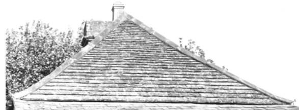
Figure 18 An alternative wind resistant hip is achieved by bedding on heavy ridge tiles supported by a hip iron at the eave. Terry Hughes
