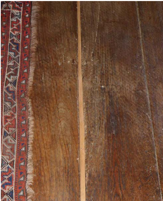
Figure 3: Gap between floorboards filled with slip of matching timber. Photo: Philip Hughes
