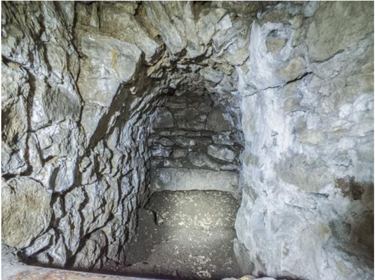
The large horizontal stone at the centre of the picture is position R2. A small part of the top of the horizontal pipe (R3) is visible in the bottom left corner.
