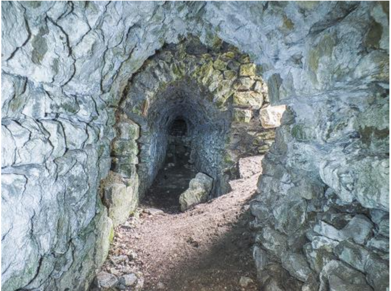
The central entrance (R5) is on the right. Again, the projecting lower arching on the right continues. It is also noticeable that the stonework on the right (south) wall is of poorer quality than the left (north) side. The gap in the arching by the entrance is also apparent.
