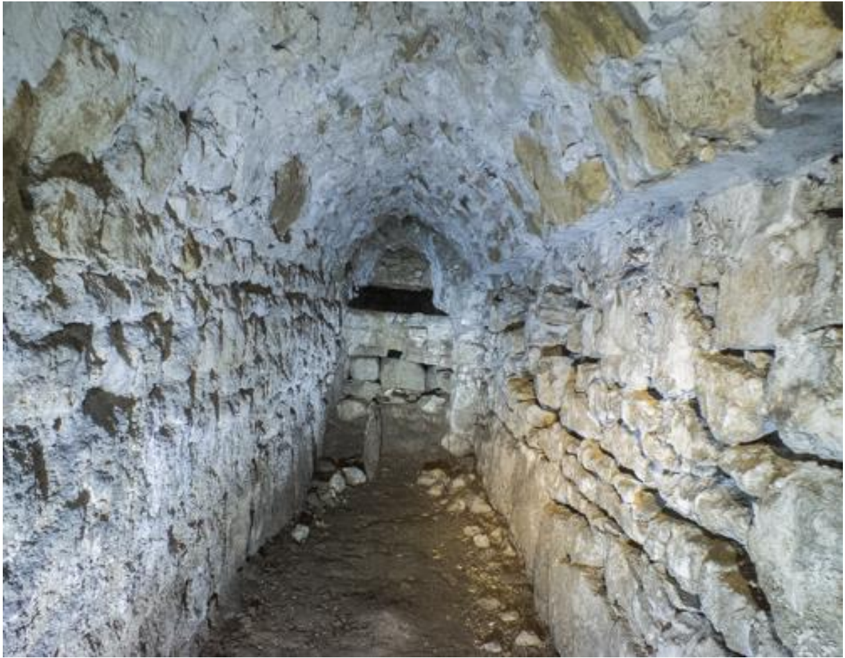
A more distant view of R3. The projecting lower edge of the arching on the right (south) can be seen running the full length of the wall.
