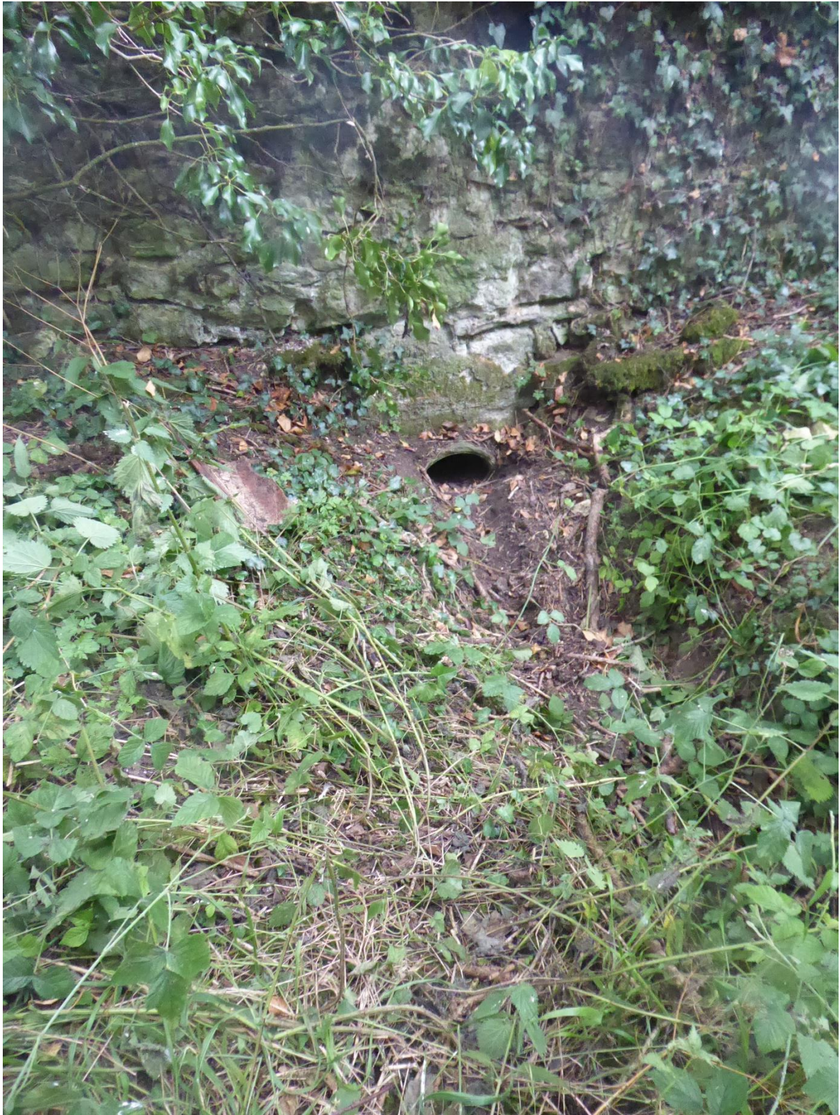
Drainage channel at SEP 5 that appears to let water in from the fields outside the wall of the abbey complex.
