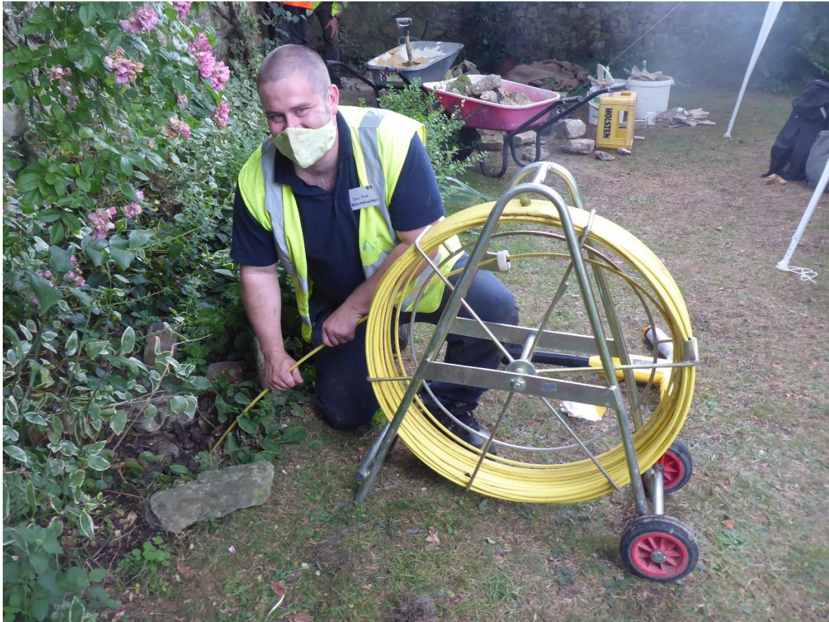
Dale Rose of Terra Measurement investigating the small drain in the current Rose Garden.
