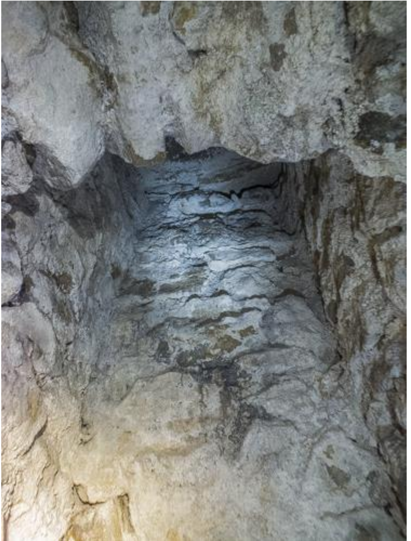
View of the broadly square cross-section shaft above the sluice through which the mechanism to lift the sluice gate would have operated.
