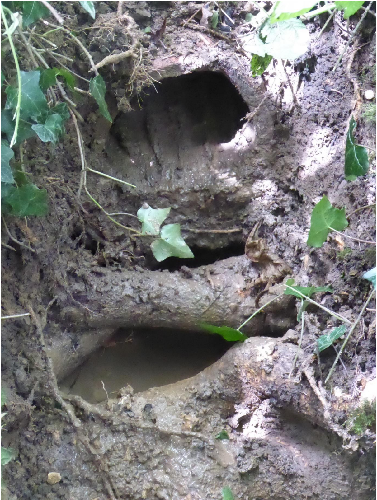
Close-up of SEP 1: Ceramic field drain at top, with water dripping through tree roots below.
