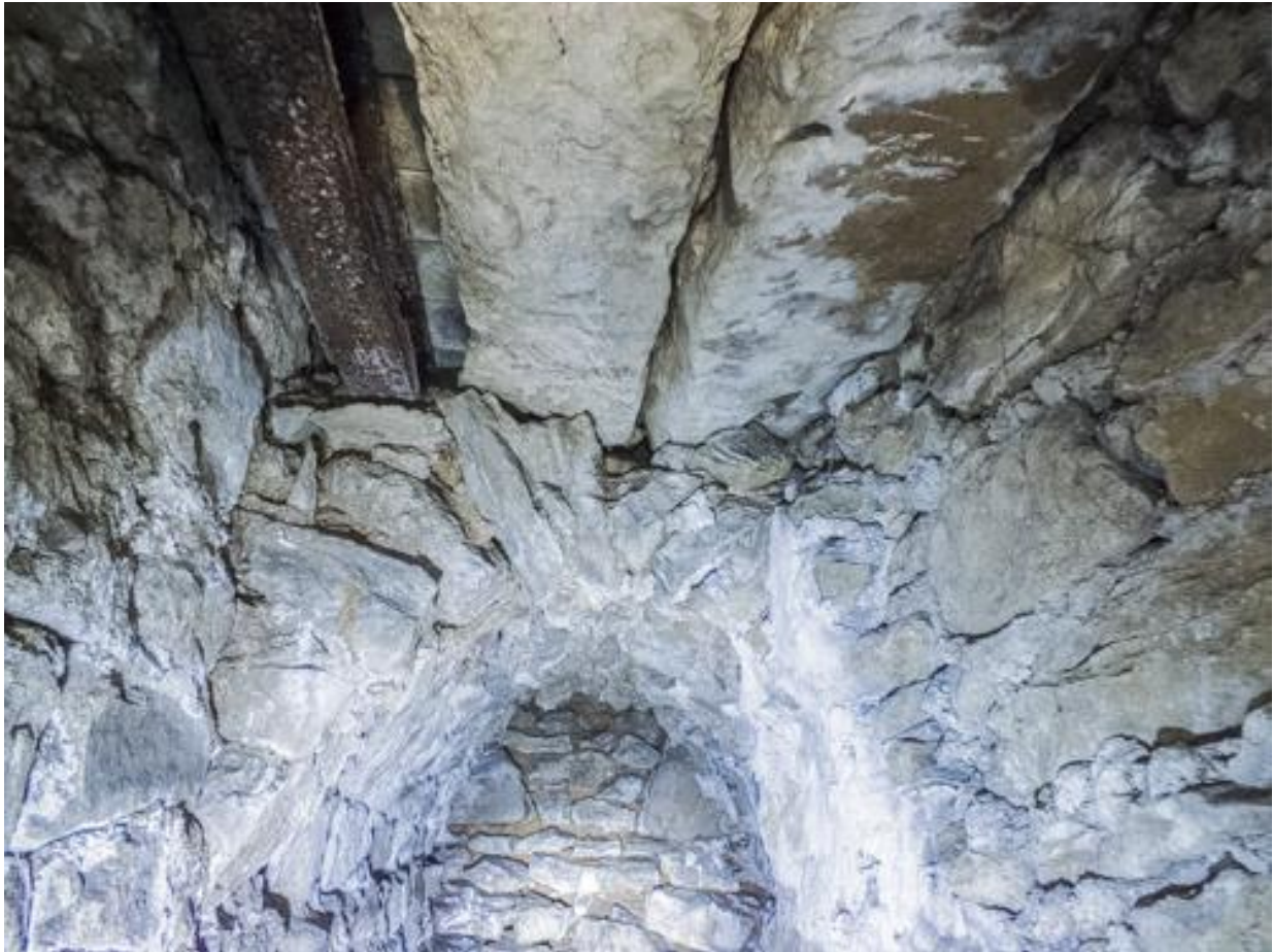
A view of the hole in the roof by the filled in east entrance.
