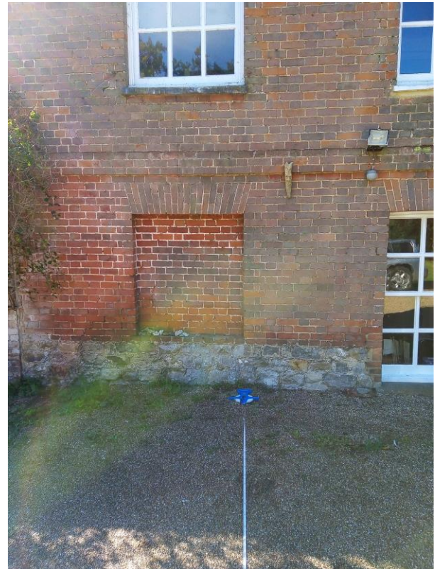
Figure 5 - Baseline reference point 'B' is situated on the western edge of the bricked up window at TQ 76105 58685.
