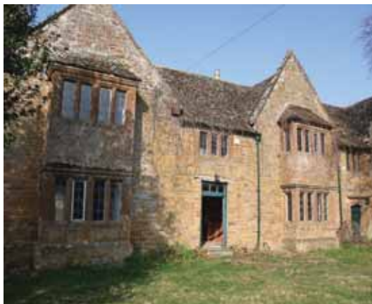
Top and above right, Grange Farm at Towersey, decayed but now the subject of repair proposals. Above, Chapter Farm, Braunston – further investigation might be necessary
