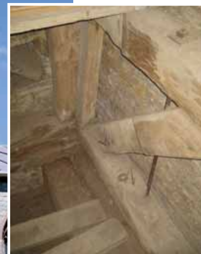
St Matthew's, Wookey, with its ancient wooden bell frame (above), in situ. The SPAB is greatly concerned by proposals to either remove much of the frame, or to relocate the bells to a new frame. The Society is keen that the frame, which is in a very good state of repair, should continue in use for the purpose for which it was constructed some 350 years ago
